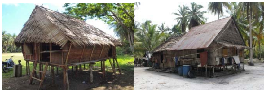
Figure 11. Leaves roof (left), and metal roof (right) on Lum's House Source: Survey, 2014
